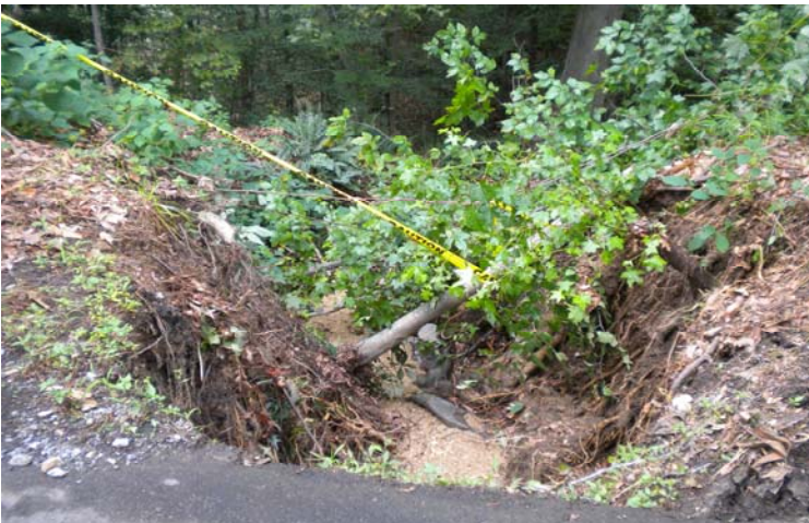
Erosion into Mill Creek from Calvert Drive due to storm water damage
