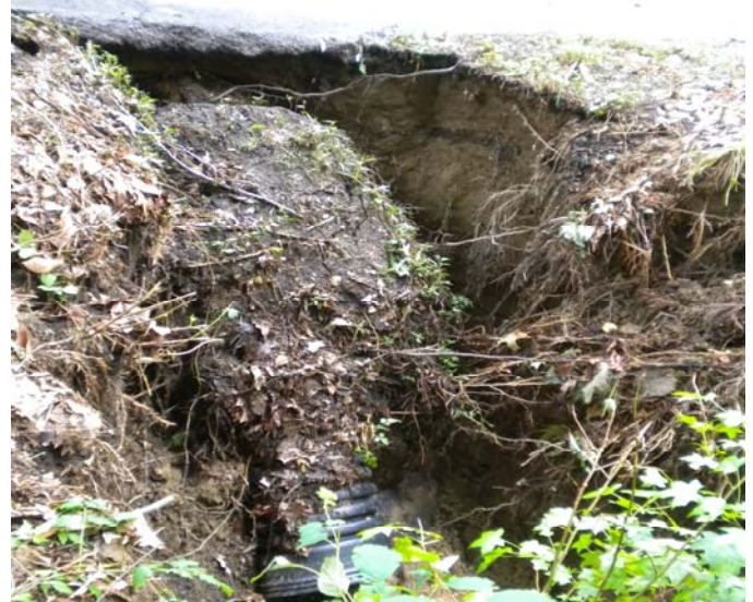
Erosion into Mill Creek from Calvert Drive due to storm water damage
