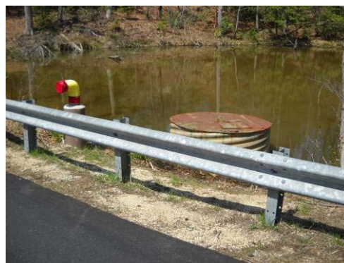
Anchor pond riser and guard rail
